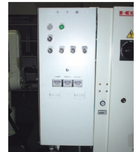
Painting unit control panel
